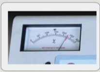
Independent Voltmeter for monitoring input line Voltage
